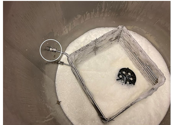
Fig. 1 A milk taxi was used for preparing and distributing milk for the calves. The location of the leaking pipe is indicated by a circle. The leak itself cannot be seen
